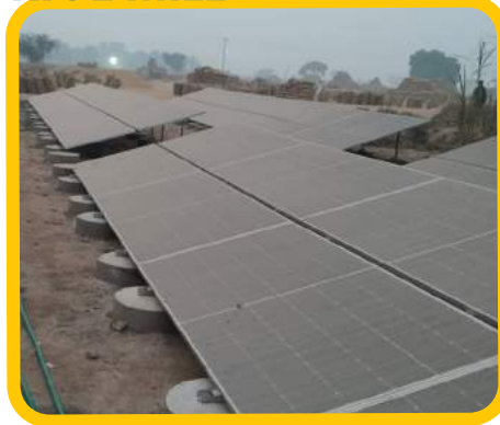
110kW Grid Tie Solar
