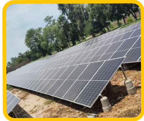
450kW Grid Tie Solar Project
