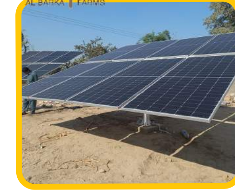
250kW Grid Tie Solar Project
