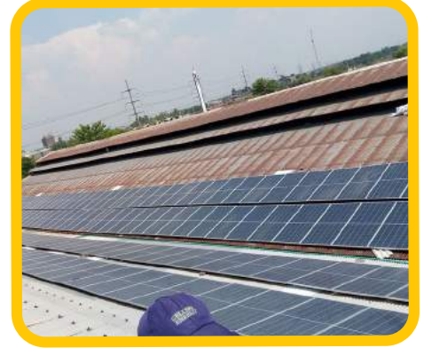
1MW Grid Tied Solar Project
