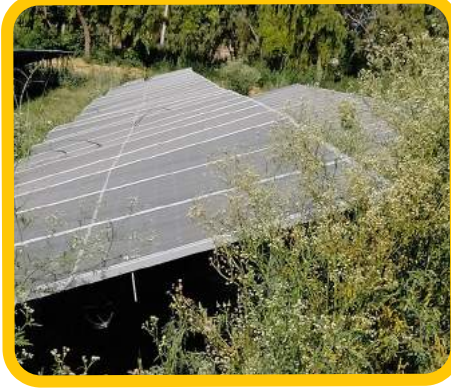
450kW Grid Tie Solar Project
