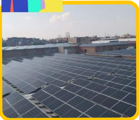
782kW Grid Tie Solar Project
