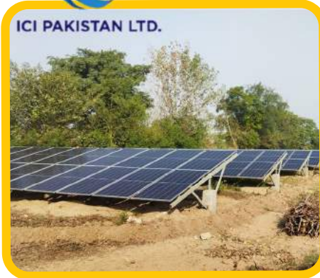
486kW Grid Tie Solar Project
