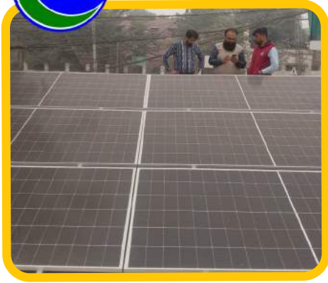
250kW Grid Tie Solar
