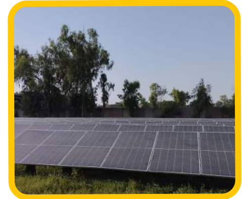
450kW Grid Tie Solar Project
