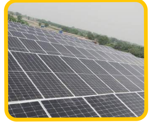
200kW Grid Tie Solar
