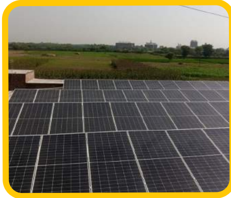
200kW Grid Tie Solar
